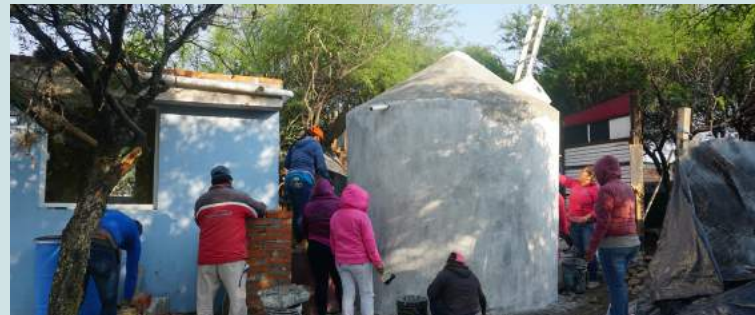
Community members build a rainwater harvesting system on a Casita Linda home in the community of Palo Colorado. In 2018, we teamed up with Casita Linda to include these systems on their home construction projects.
